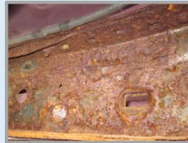
Complete Surface Rust with Descaling
