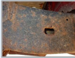
Light to Moderate Surface Rust
